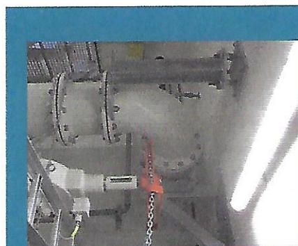
Remedie: extra steun horizontale persleiding.
